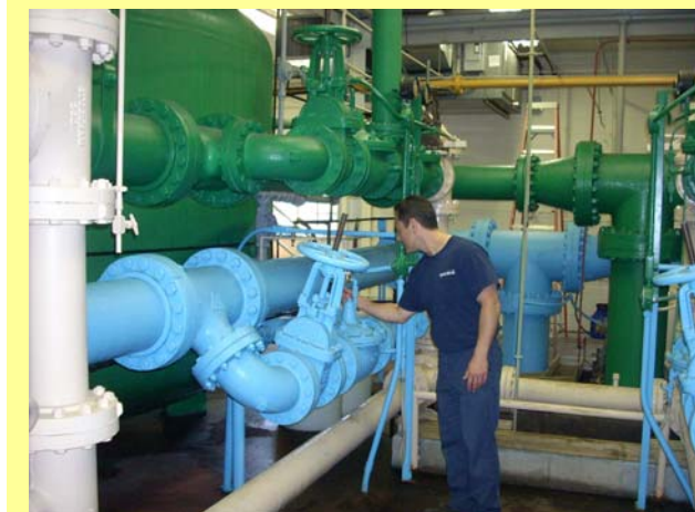
Treatment and Pumping Apprentice Operator backwashing manganese removal filters at the Black Brook Water Treatment Plant in Whippany
