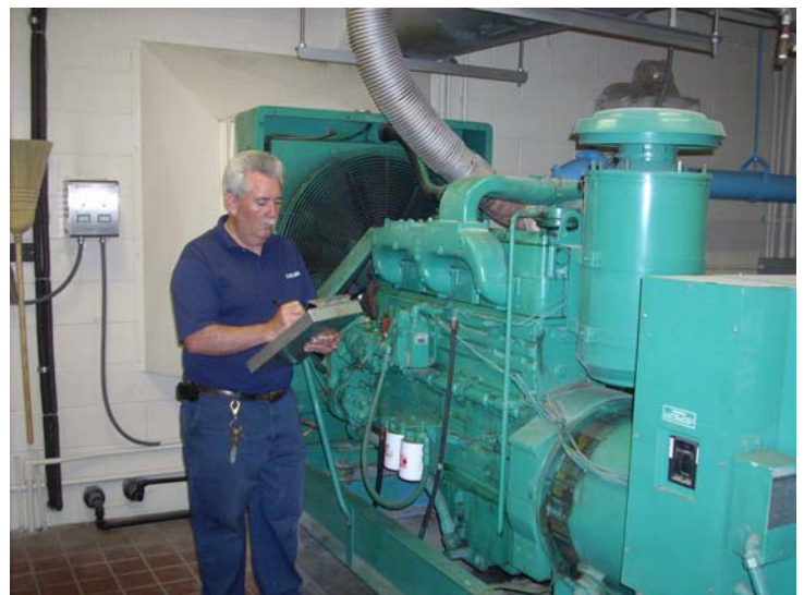
Treatment and Pumping Operator checking emergency power generator at Countrywood Booster Station in Cedar Knolls
